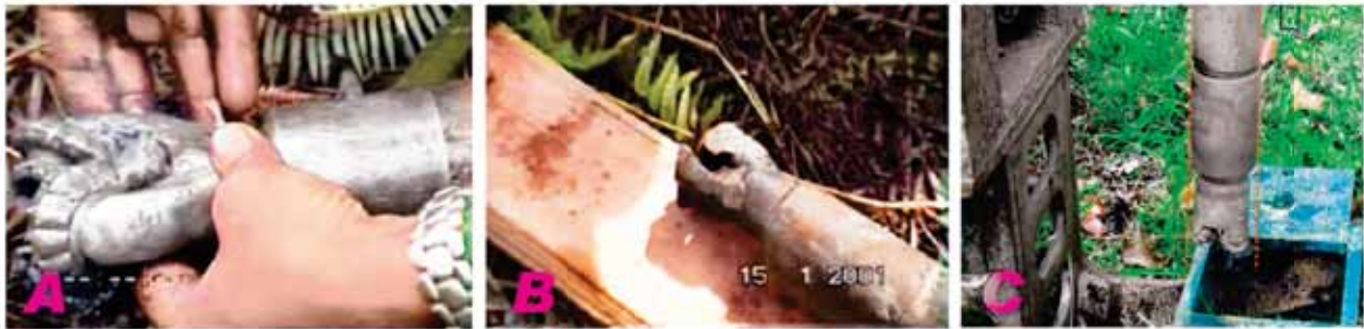
Figure 12a: Different soil type require different cutting bit, and cutting bits vary from simple wings to spiked rollers. (A) Roller bit with compatible rod but used in wrong soil type. (B) "Dragbit" being passed off as roller bit. (C) Correct soil type, acceptable rig but roller bit smaller than drill string.
